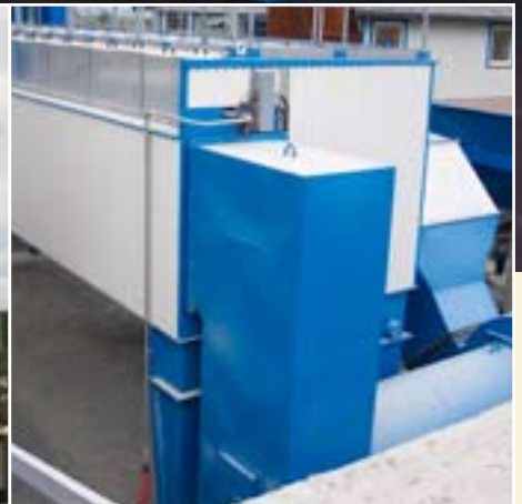
Exhaust Gas Ducting
