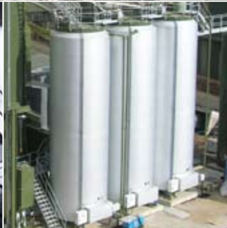
Vertical Bitumen Tanks
