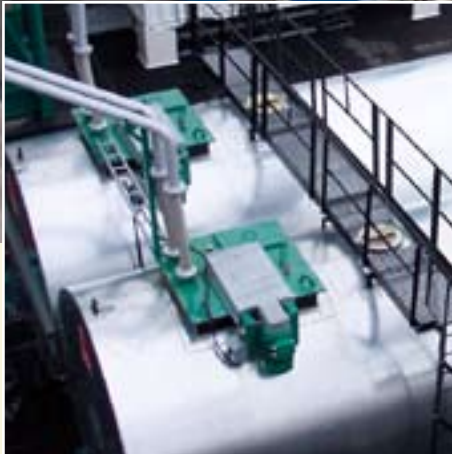
Horizontal Bitumen Tanks
